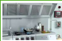
Commercial Kitchen Suppression Systems
